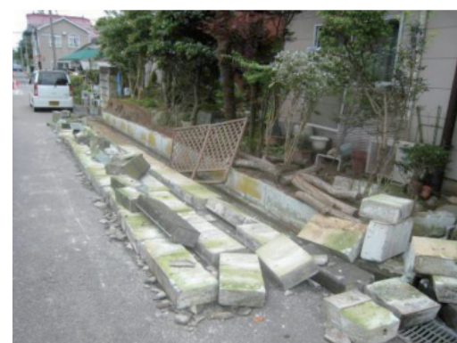
Collapsed stone wall
