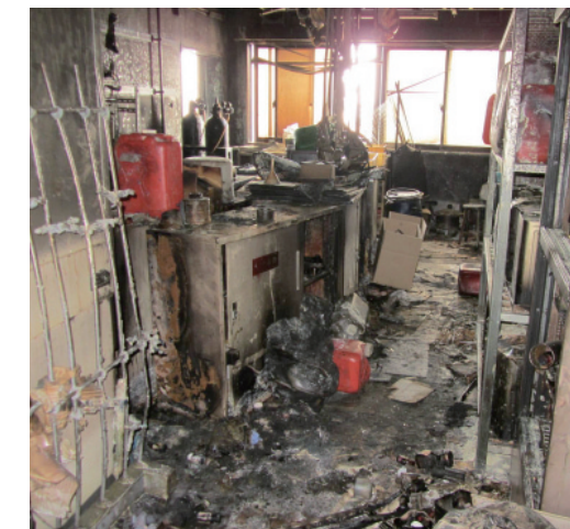
Traces of a fire of a chemical laboratory due to the shaking (in Tohoku Univ.)
