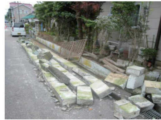
Collapsed stone wall
